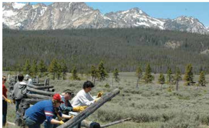
Youth helping to replace obsolete fencing to enable antelope passage – a rewarding day of work!
