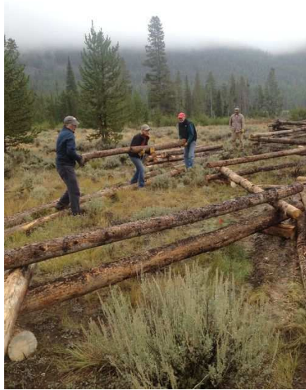
Sawtooth Society board and members worked together to build a beautiful logworm fence to protect Pole Creek. Photo by Kelly Conde
