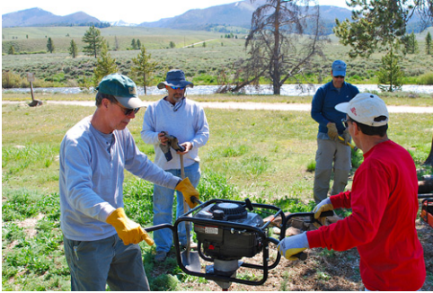
The “Jersey Boys” traveled across the country to decommission old hitching posts, build new ones and refurbish feeding troughs at several trailheads.
